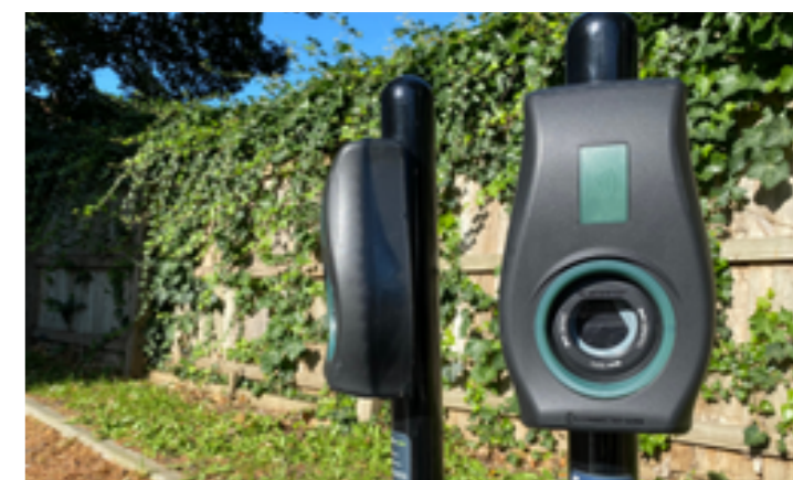
A total of 103 EV charging points were installed in 26 car parks across the district.
